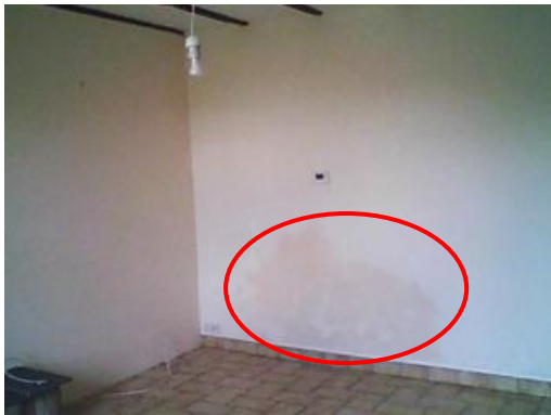
Visual evidence – damp stain (circled red).
